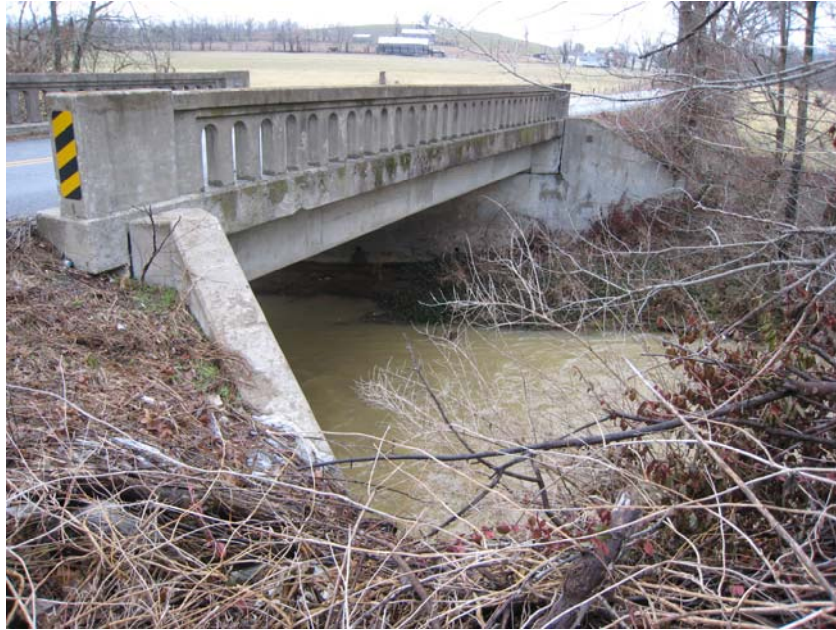
Figure 6: Bridge after a Rain Event
